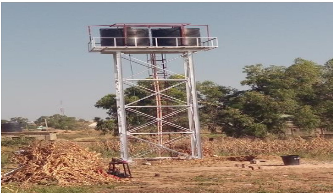
Figure 1: Provision of motorized borehole with overhead tanks in Lagos State
