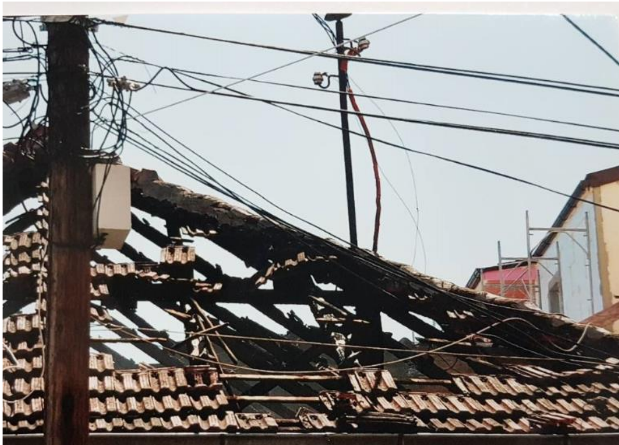
Figure 2. Damaged roof where is found source of fire
