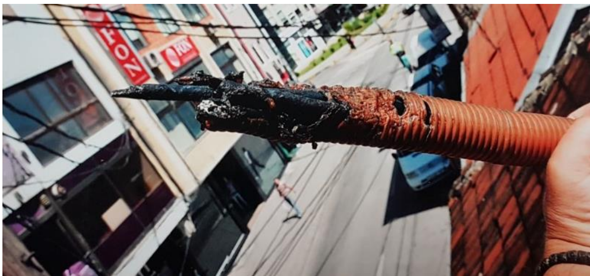
Figure 1. A burnt conductor as a result of a short circuit
