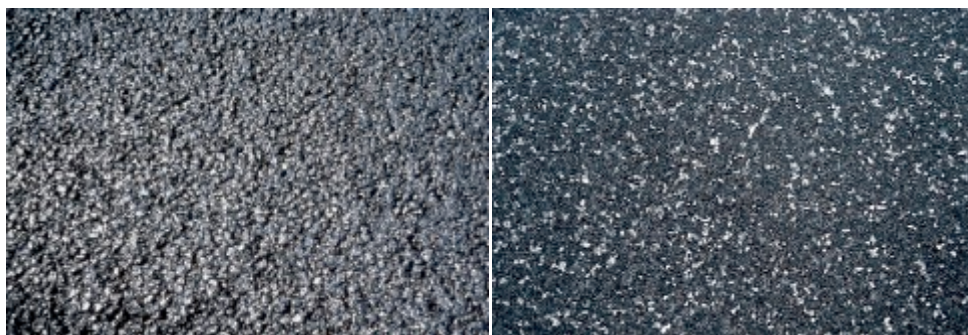
Figure 15. Non-blunted (left) and blunted (right) surfaces of Stone Mastic Asphalt wearing courses [DAV 2000]
