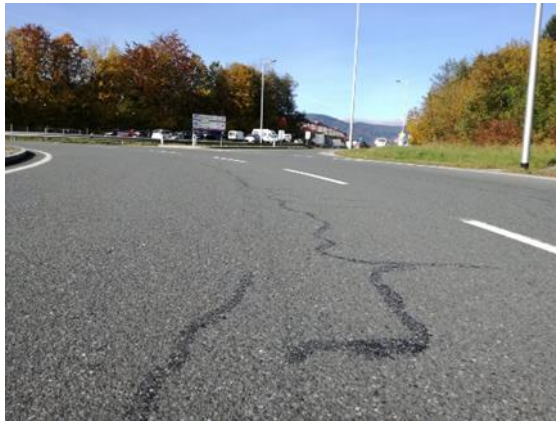
Figure 9. Irregular longitudinal and transverse cracks (Hrapović 2020)
