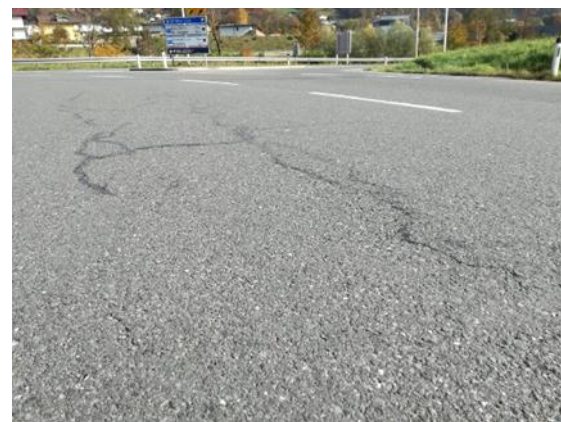
Figure 12. Alligator cracks partially repaired with hot bitumen compound, exit area on B154 Mondsee (Hrapović 2020)
