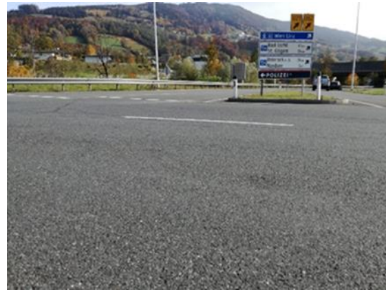
Figure 10. Plucking, transverse crack (Hrapović 2020)
