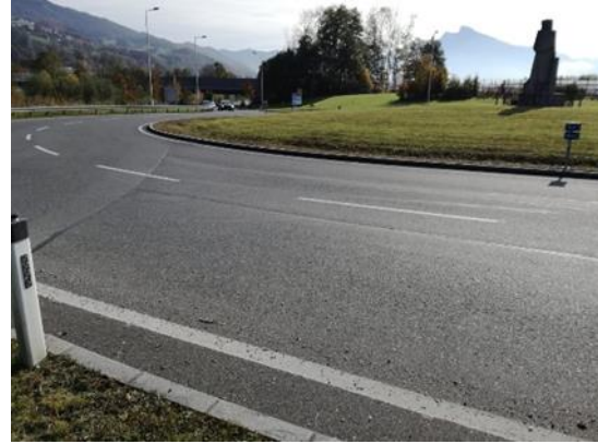
Figure 18. Continuous transverse seam crack (construction joint) (Hrapović 2020)
