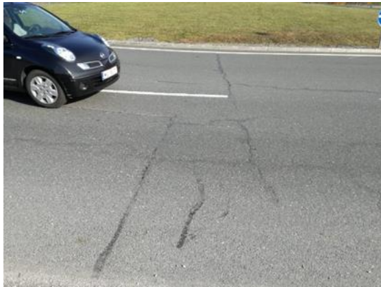
Figure 13. Longitudinal and transverse cracks (Hrapović 2020)
