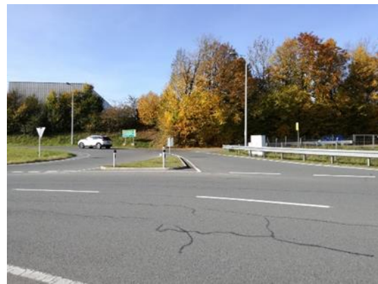
Figure 16. Irregular longitudinal and transverse cracks (Hrapović 2020)
