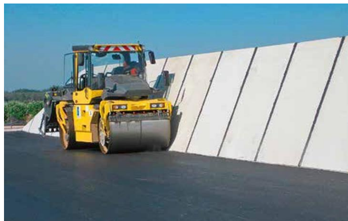
Figure 6. This must be done precisely up to the edge and compacted. (Müller 2014)
