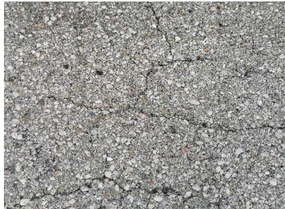
Figure 9. Cracks in asphalt as a result of low temperature
