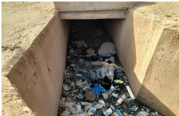
Photo 4: Blocked gutter at Boundiali market
