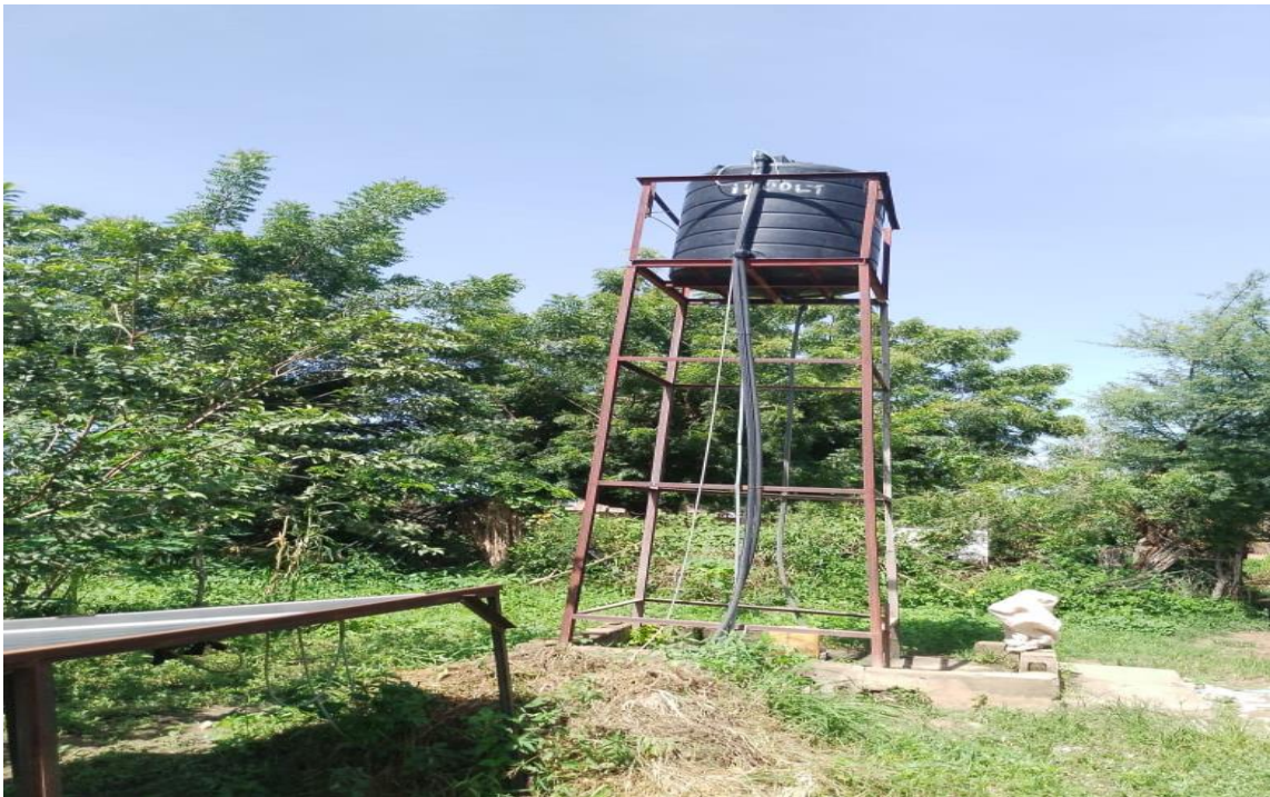
Photo 4: Water tower connected to a borehole in the "Dèmèton" market garden area
