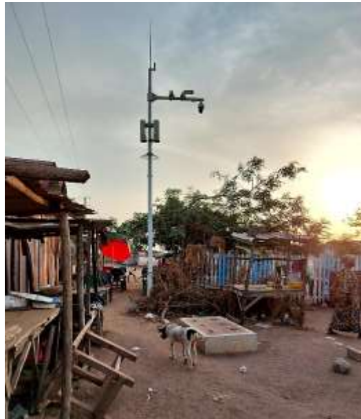
Photo 3: Installation of surveillance cameras at the entrance to the courtyard of a resident
