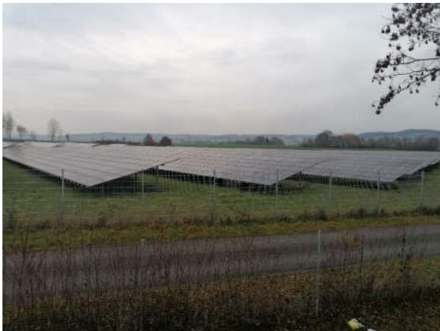
Figure 3: PV plants next to the highways in Germany (Hrapović, 2023)
