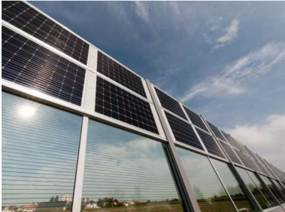
Figure 4: Photovoltaic system on a noise barrier (Vielhaber, 2021)
