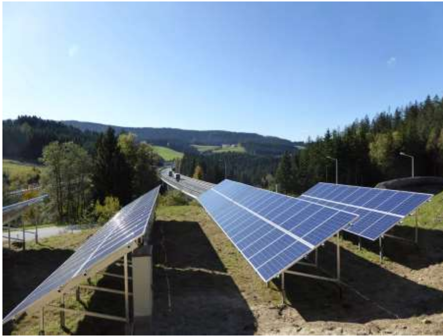
Figure 2: Photovoltaic system at the Herzogberg tunnel, A2 South motorway (Vielhaber, 2021)
