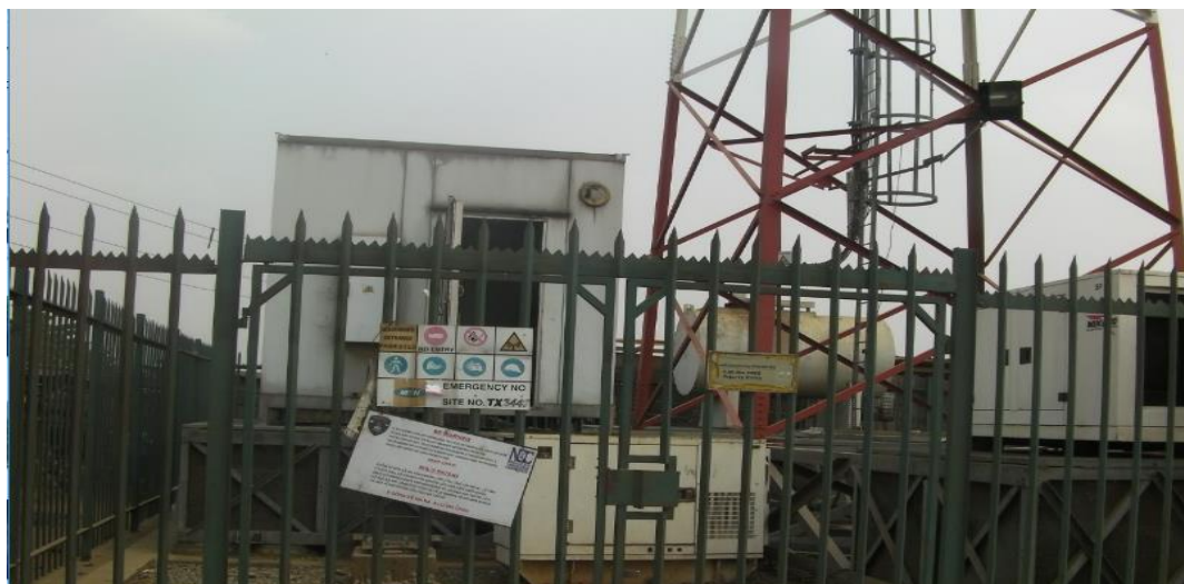
Figure 2: Isolo base station in Akure, Ondo State
