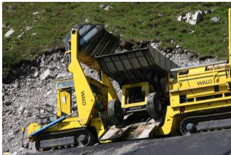
Figure 14. The mixture is tipped into the gutter at the front of the paver winch train and then transported via the driver's cab into the paver feed wagon (Danklmaier, 2008)
