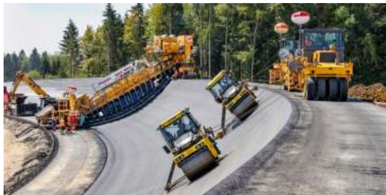
Figure 21. The exact compaction of the parabolic surfaces is done by specially shaped rollers 3
