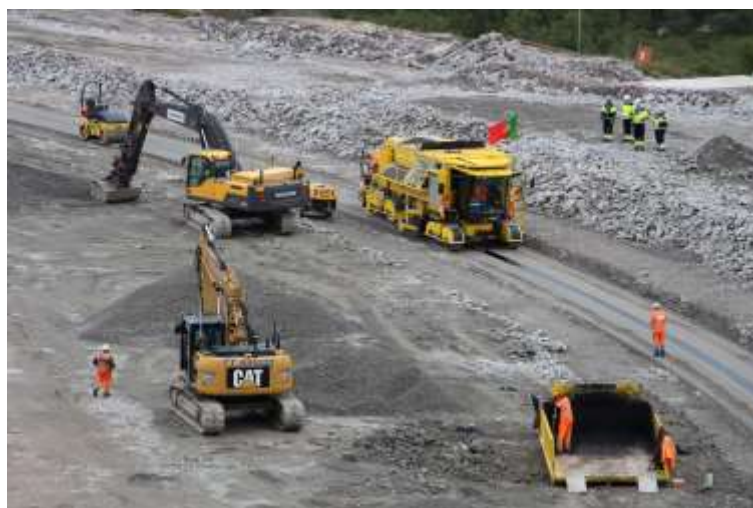
Figure 9. Installation of the asphalt core seal on a dam for a hydroelectric power plant in Norway 1
