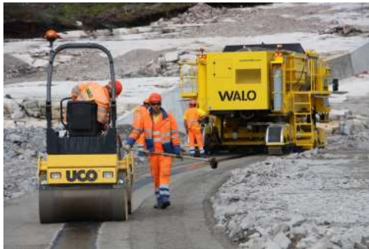
Figure 10. Installation of the asphalt core seal on a dam for a hydroelectric power plant in Norway 1
